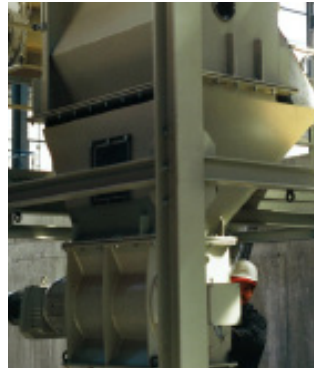
Partial view of ZZ-Separator SepK12/250-4 Separation of PUR of crushed refrigerators
